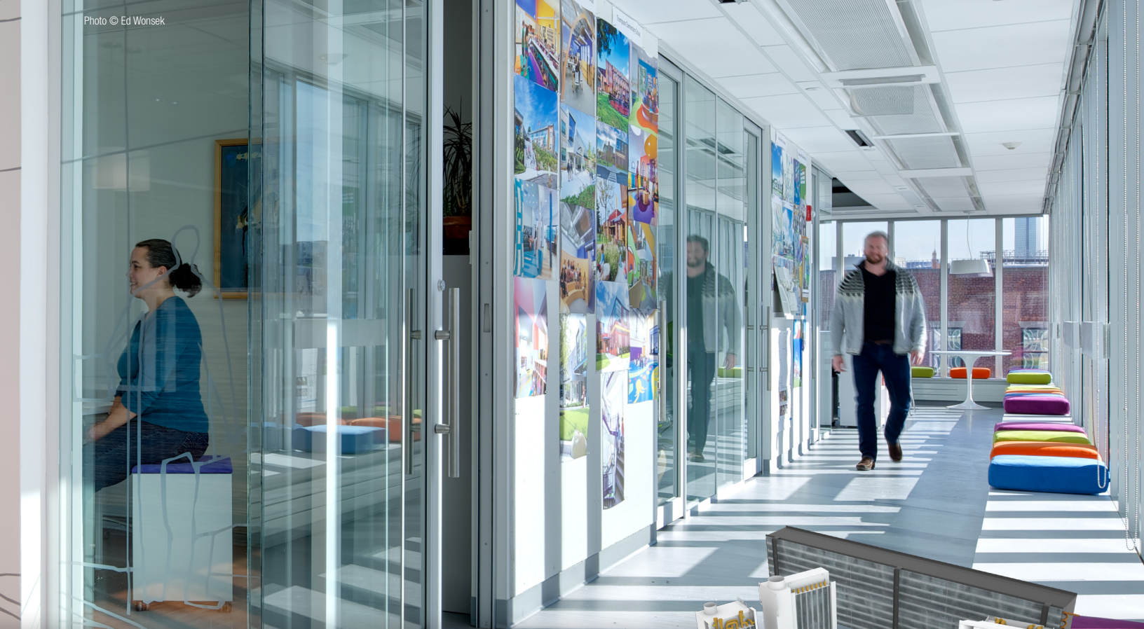
Above: Chilled Beams
